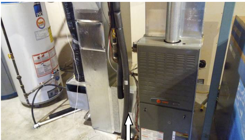
Heating coil from CHP into the furnace
