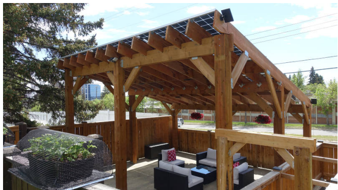
1. A solar pergola with translucent solar modules.
