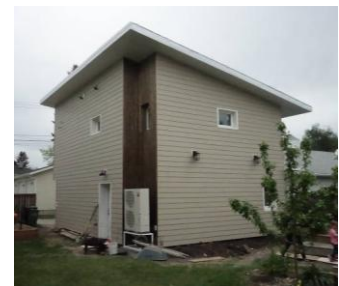
3. A Cold Climate air source heat pump unit on a garage suite.
