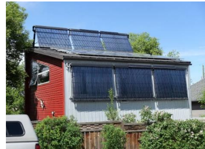
5. Solar thermal collectors for domestic hot water and hydronic heating.
