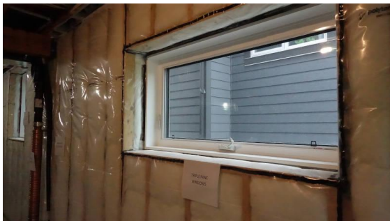
6. An example of double stud walls and triple pane windows in a basement
