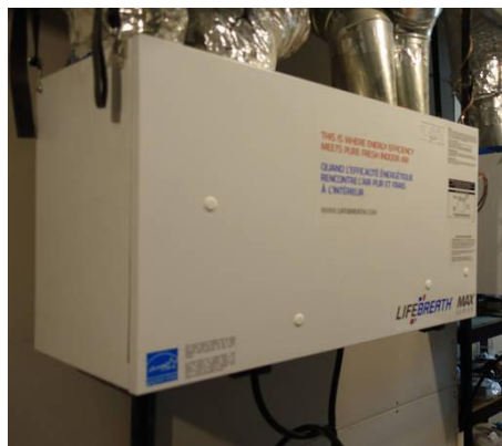
8. A heat recovery ventilator (HRV).
